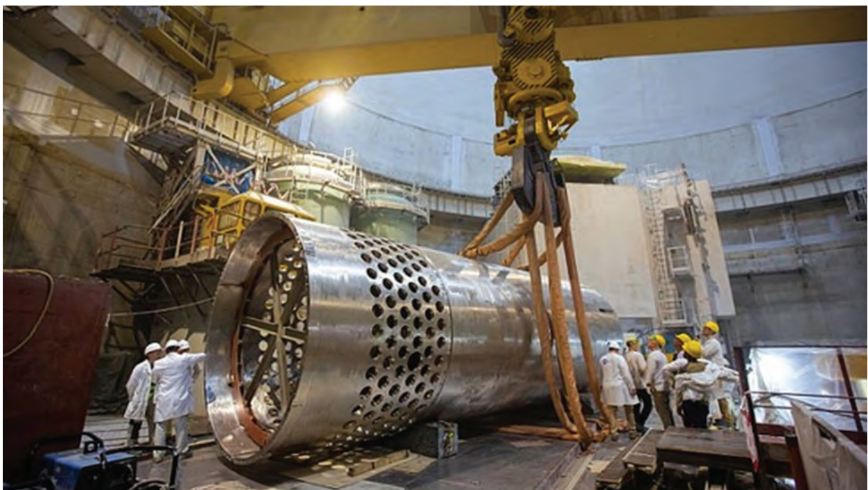
Work to install Rooppur 1's core barrel was completed in May 2023 (Image: Rosatom)
